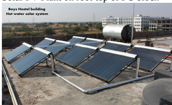
Solar water heating system on Boys hostel
