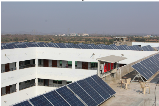
Solar PV Plant on roof top of PG block
